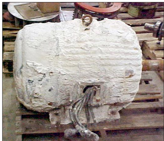
Figure 15. Motor with blocked cooling fins.
