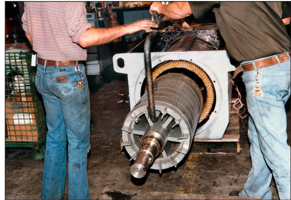
Figure 17. Rotor removal using a rotor removal tool.
